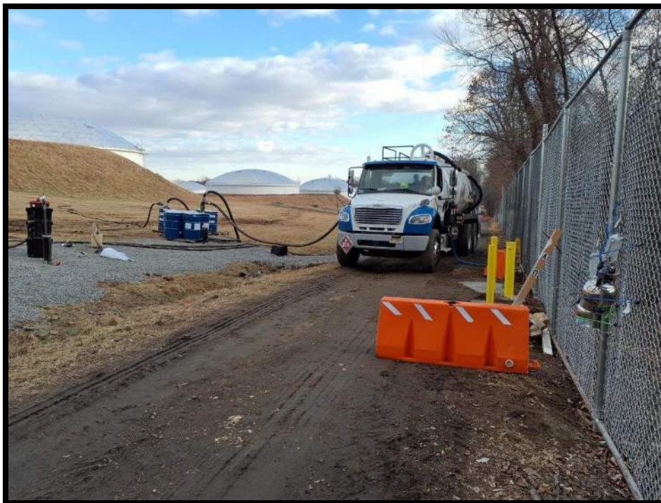
Photo of monitoring location AA-3 (Summa canisters connected to fence on right) relative to LNAPL recovery operations (vacuum enhanced fluids recovery, VEFR).
