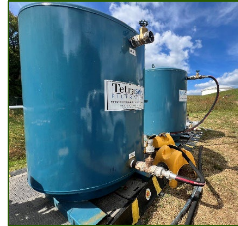
Water Treatment System
