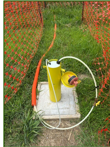
Examples of On-Site Monitoring Wells
